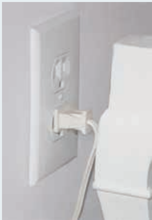
Damaged power supply cord
